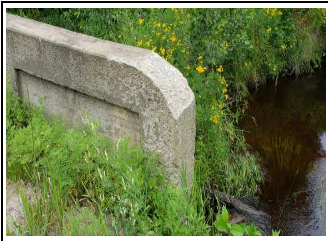
Photo 8 Moderate scaling noted on substandard traffic barrier
