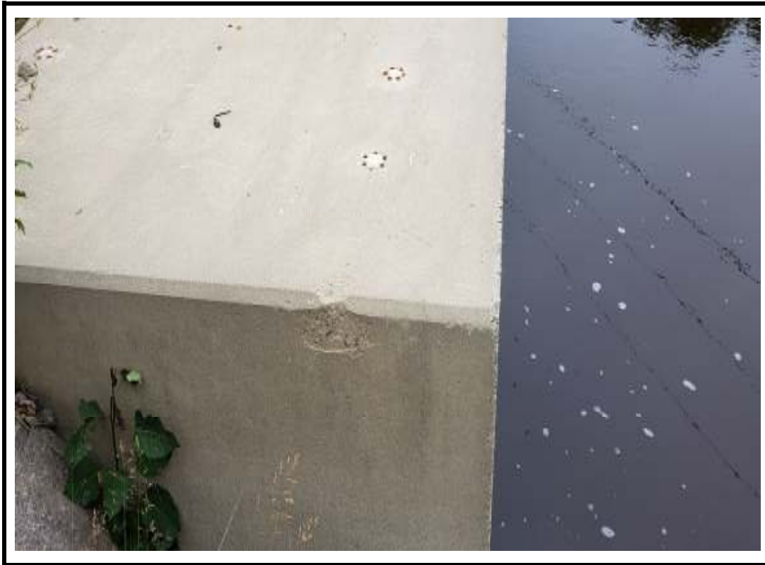
Photo 9 Spall noted on exterior interface of vertical leg and soffit
