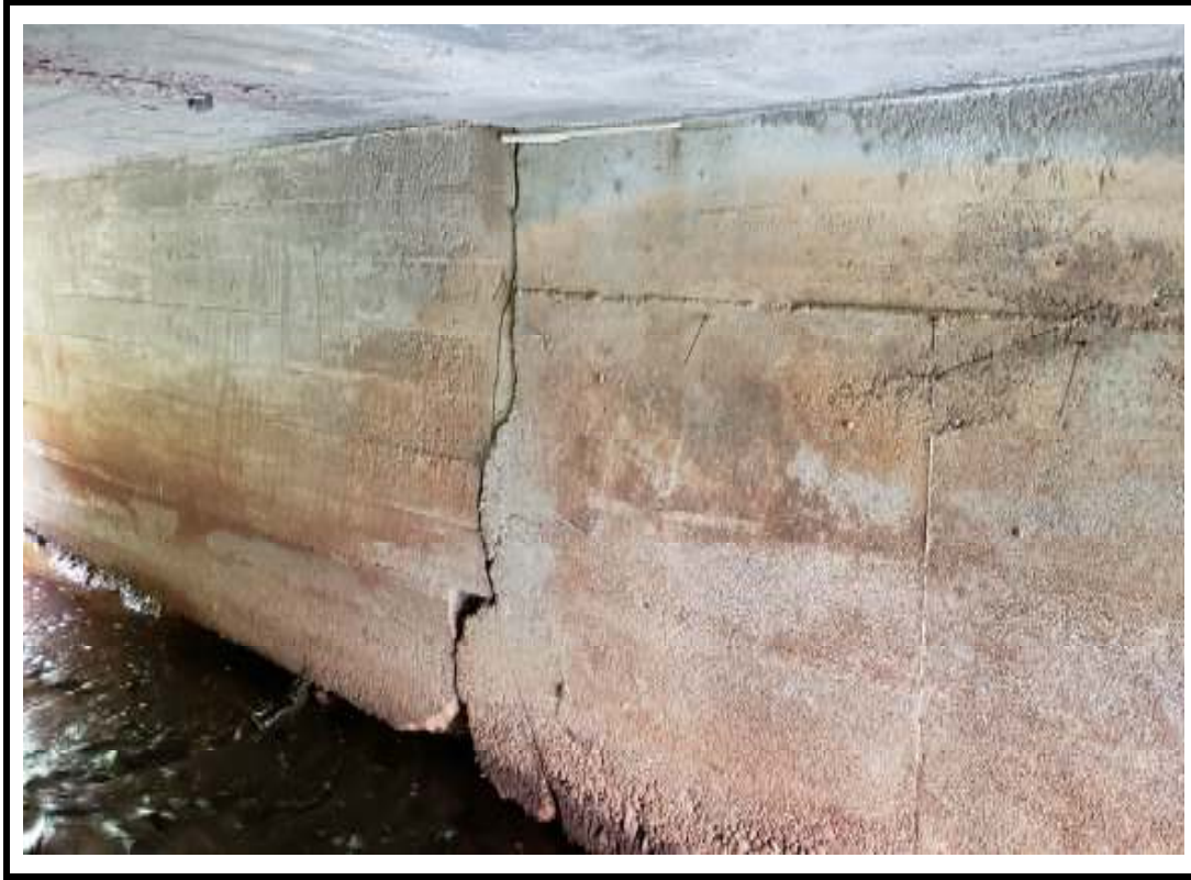
Photo 11 Full length crack and undermining noted on west abutment wall
