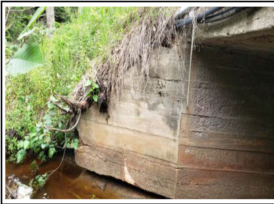
Photo 15 Moderate honeycombing, and undermining noted on southwest retaining wall
