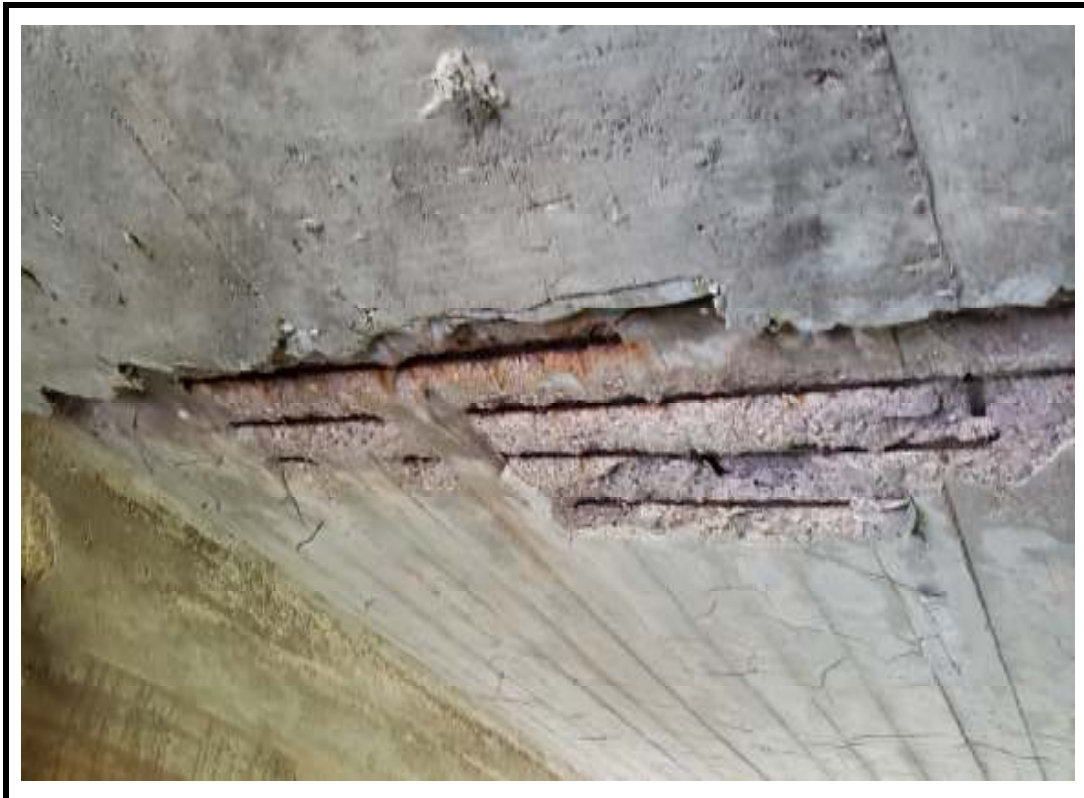
Photo 12 Large spalls with exposed corroded reinforcement noted on soffit at mid span
