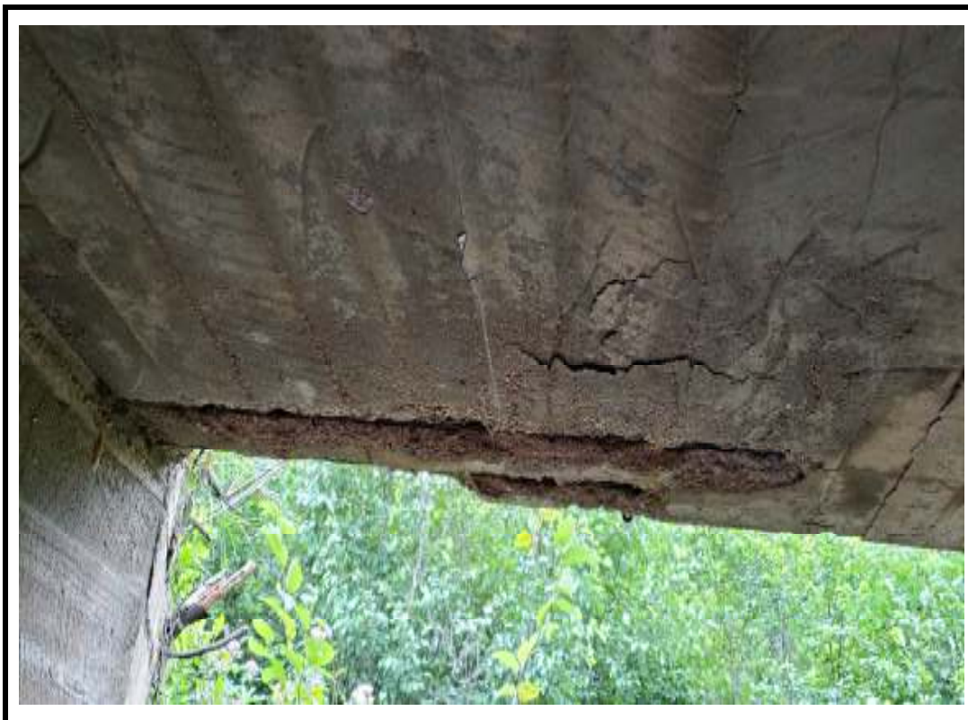
Photo 14 Delamination and spalls with exposed corroded reinforcement noted on soffit at south end
