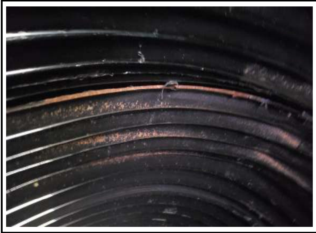
Photo 9 Light corrosion noted inside barrel at joint
