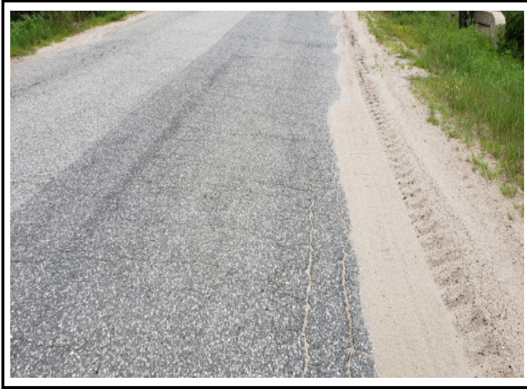
Photo 7 Horizontal and vertical cracks with tire rutting noted on wearing surface throughout
