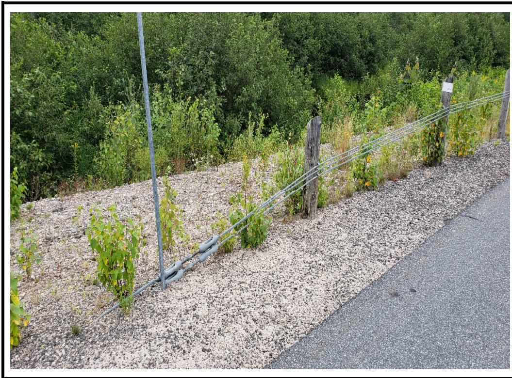
Photo 6 No end treatment present at the time of inspection
