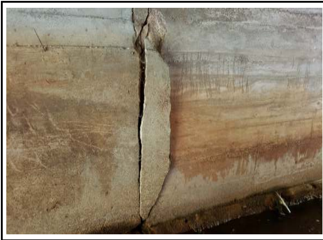
Photo 13 Large spall with portion coming out at construction joint on east abutment wall
