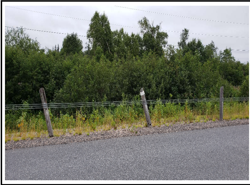
Photo 7 Barrier posts leaning at northeast approach
