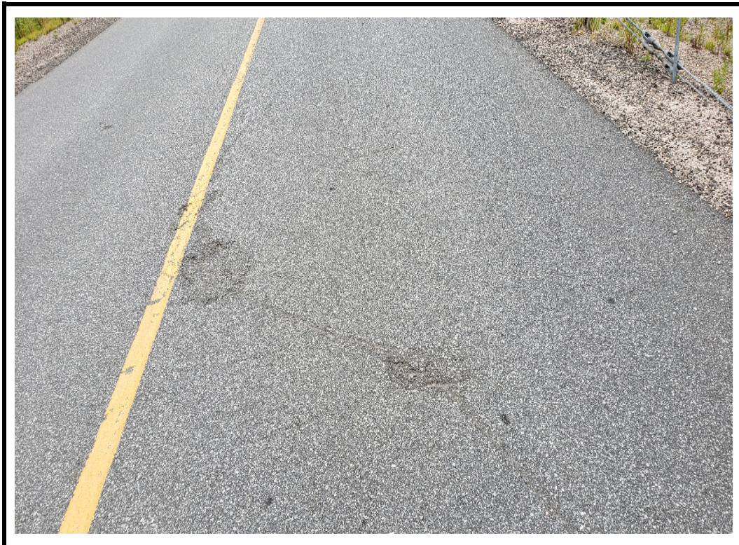
Photo 8 Potholes and previous repairs noted on west approach wearing surface
