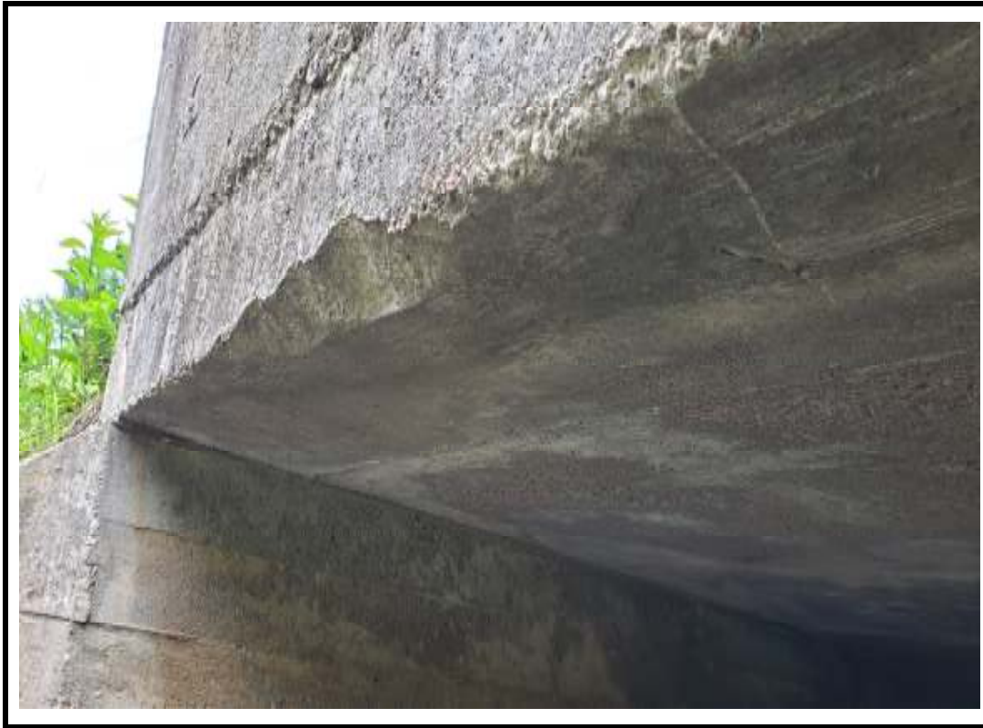
Photo 9 Spall noted on soffit at north end
