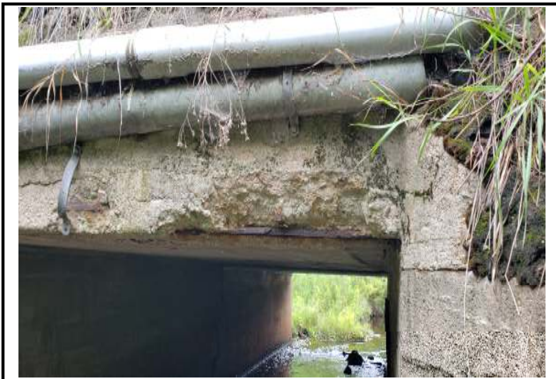
Photo 16 Large spalls with exposed corroded reinforcement noted on south fascia
